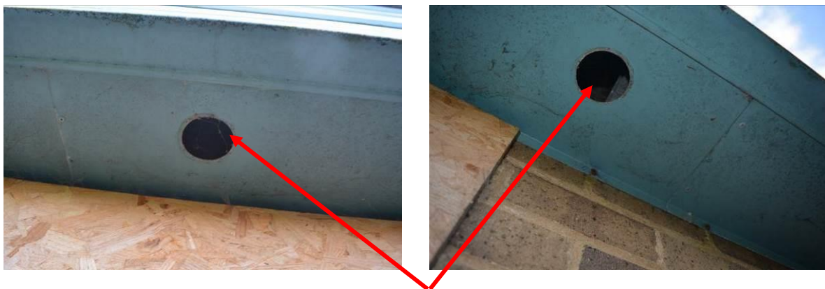
Figs. 15 & 16 External gaps / vent holes (arrowed)
