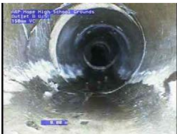
UNKNOWNX_e0e87def-a566-4820-bfd2-1157fa7d0d86_2021 1125_095407_250.jpg, 00:00:03, 0.22 m Cracks, multiple at joint from 7 o'clock to 5 o'clock
