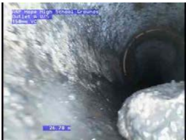
UNKNOWNX_f373b58d-0d7d-4065-9837-d61e995b3a87_202 20110_081840_276.jpg, 00:02:45, 26.79 m Settled deposits, coarse, 15% cross-sectional area loss, Brick
