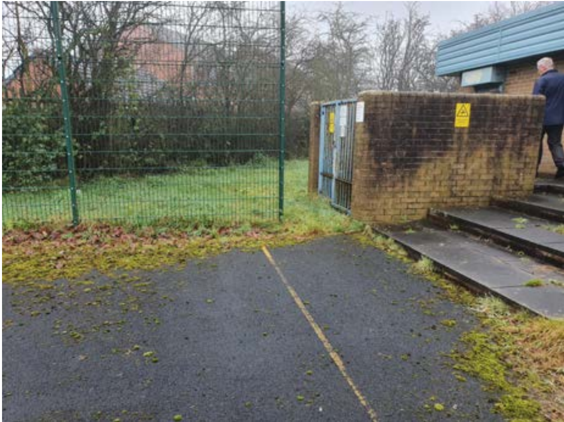
Photograph 5: Sub-station present to the southwest of the school.
