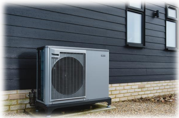
Air Source Heat Pump - External Plant
