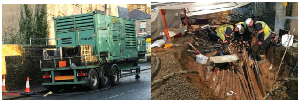
Figure 3-24: Response required due to substation flooding 23
